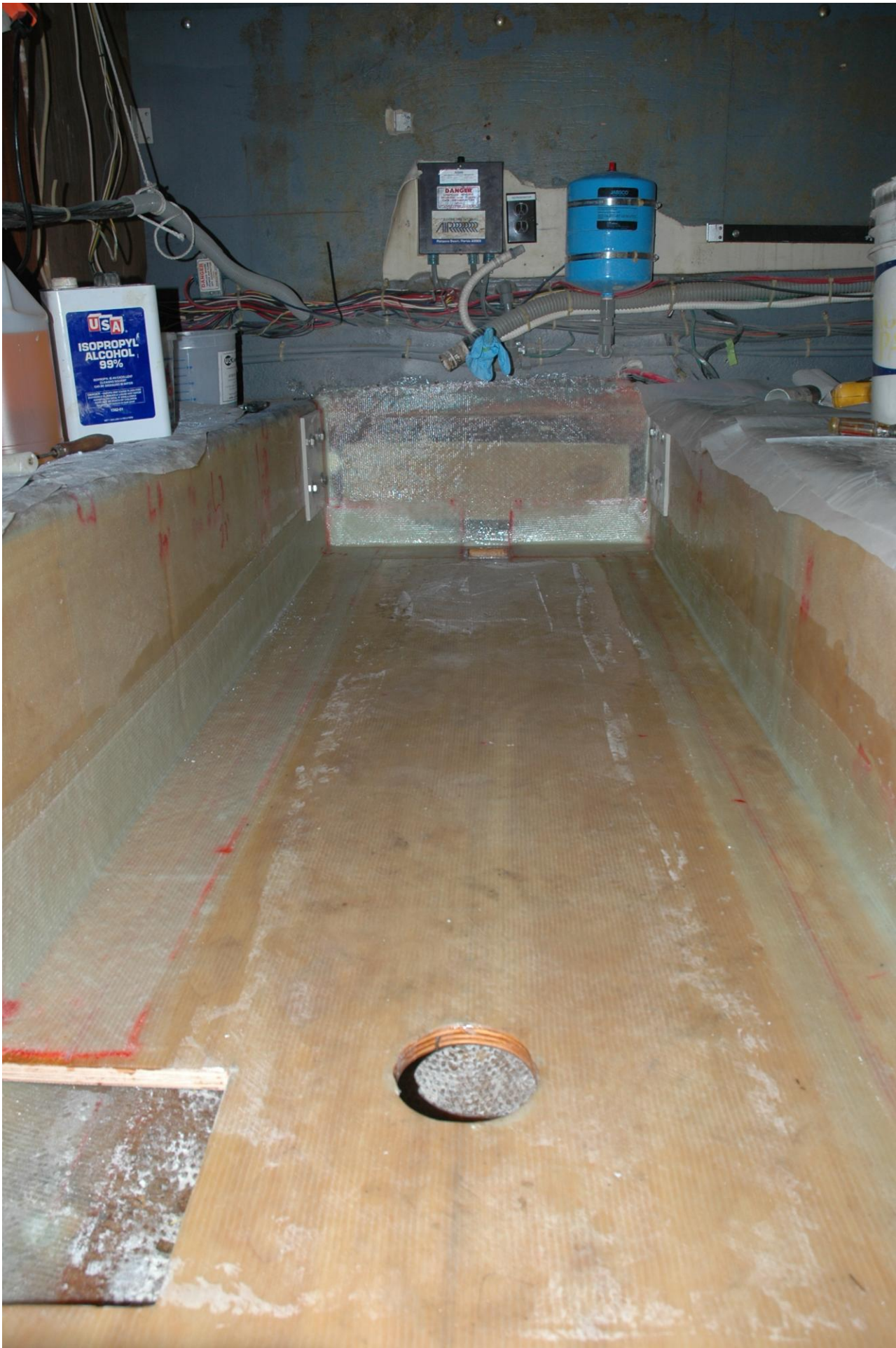
Figure 26 After a month in the bilge I have new stringers completely encapsulated in epoxy and glass.
