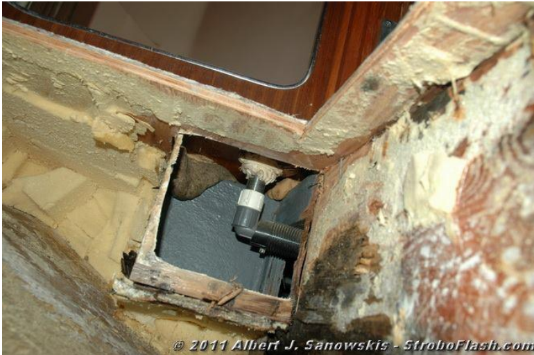
Figure 7 Shower Drain revealed
