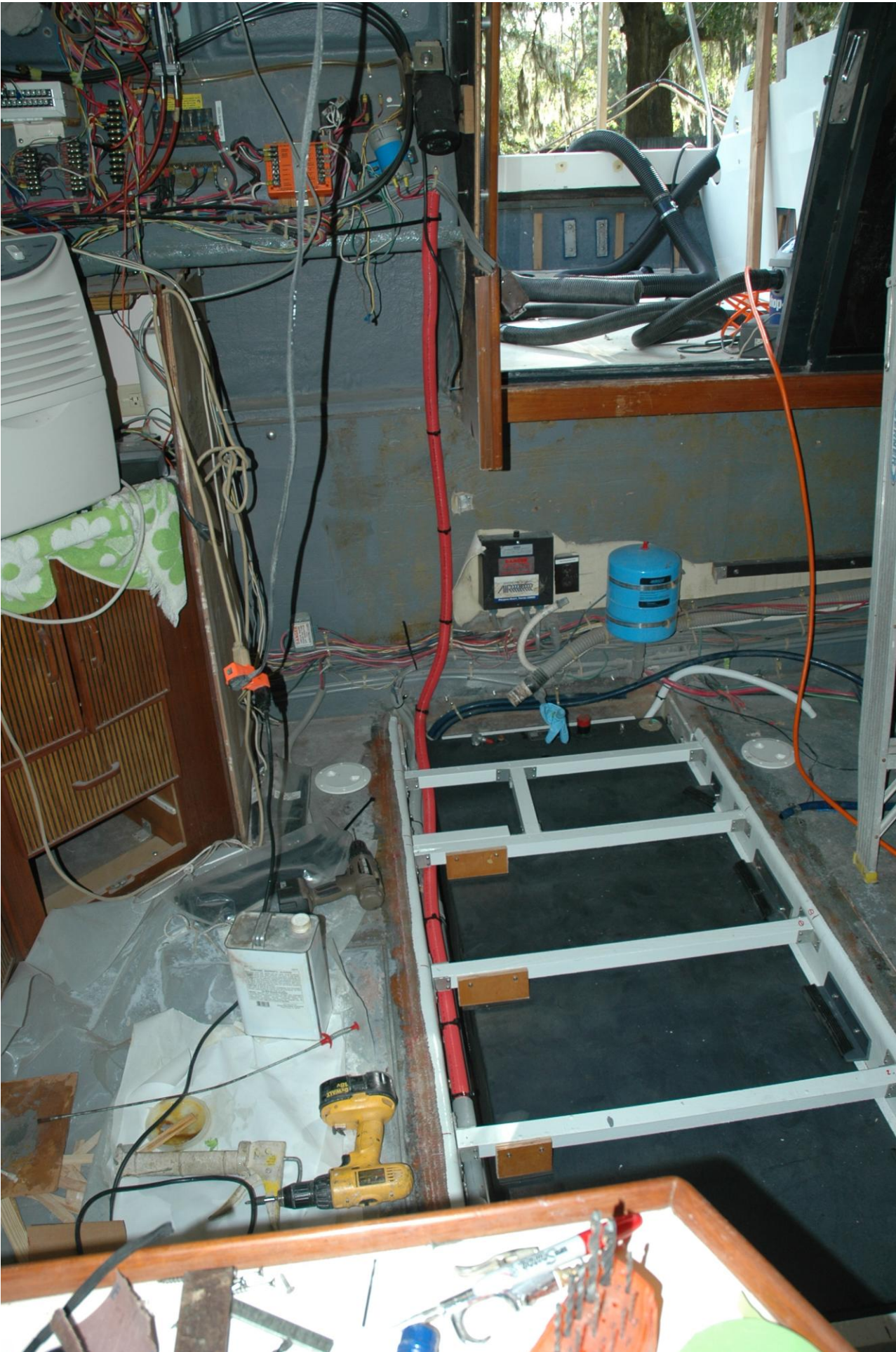
Figure 28 The new .125" wall 5052 aluminum water tank installed and resting on 1/4" rubber strips. The tank is coated with coal tar epoxy for maximum corrosion resistance.
