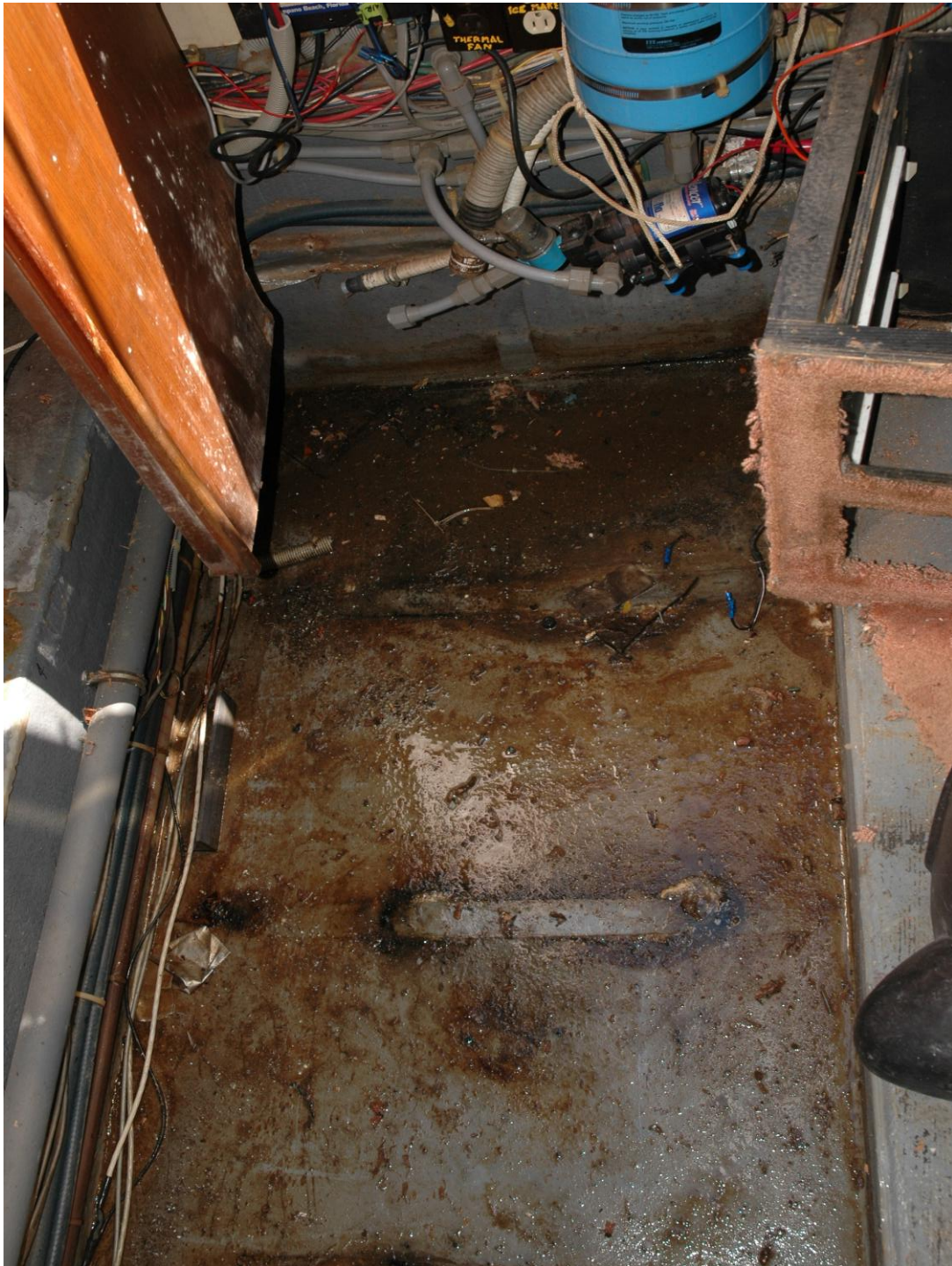
Figure 20 This is the wet mess I found under the water tank. The tank had a zillion holes in it from crevice corrosion. Google it.
