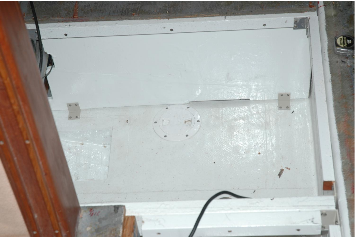
Figure 29 I also installed a 6" inspection hatch so I can see inside the bilge under the water tank just incase any water might get in there. I can't see how but just in case.
